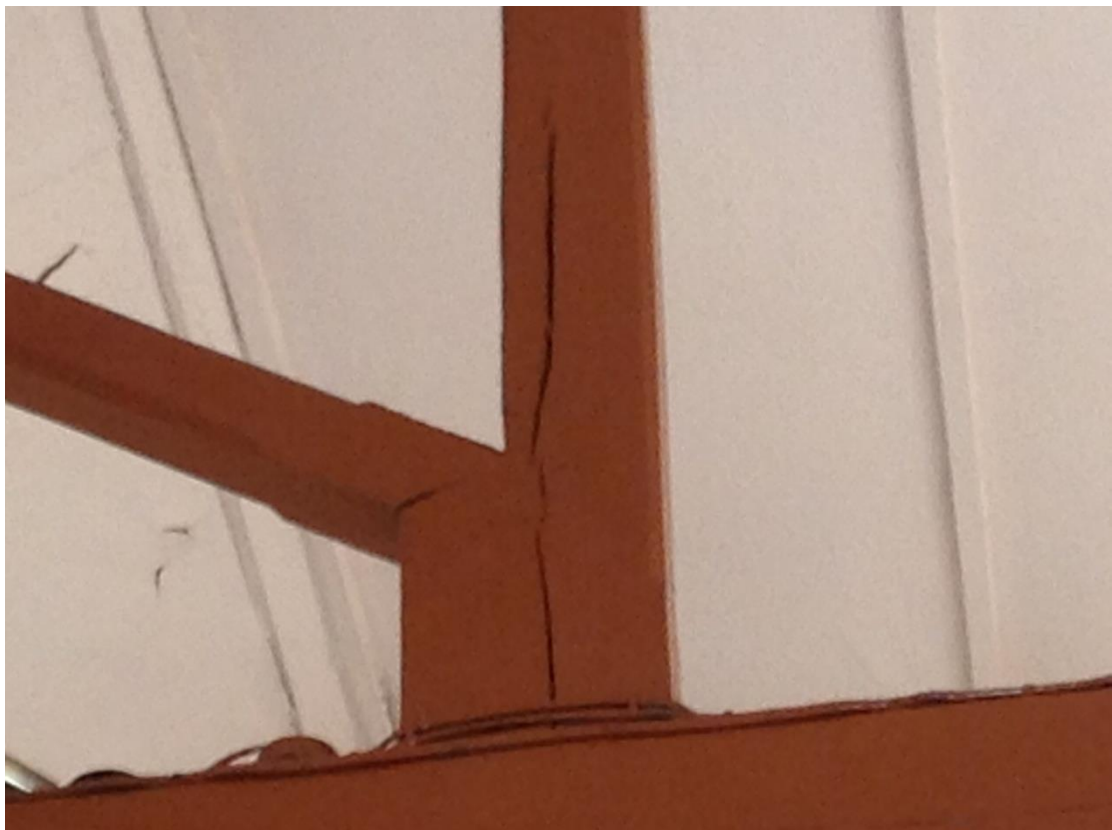
Image 7: Shows roof joist supports cracking.
