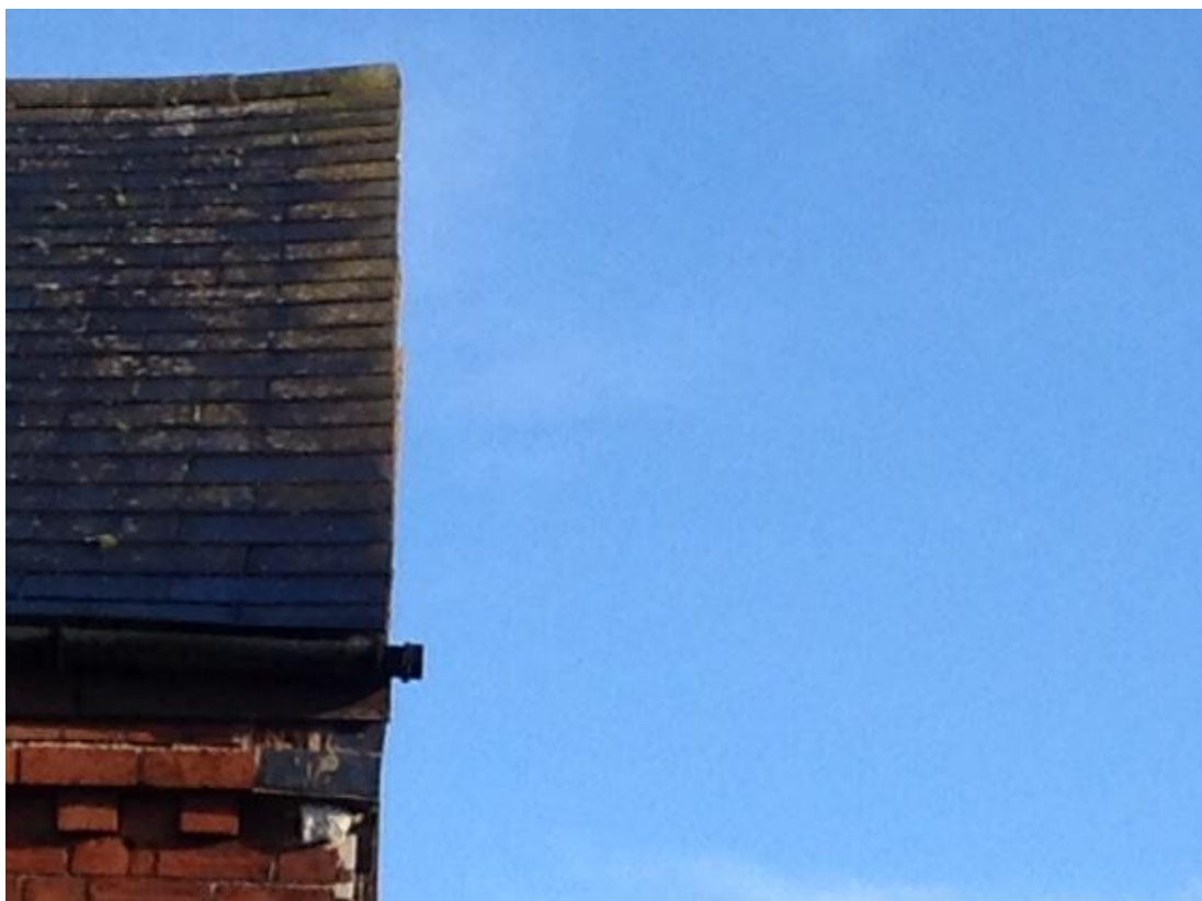
Image 9: End gable showing signs of movement.
