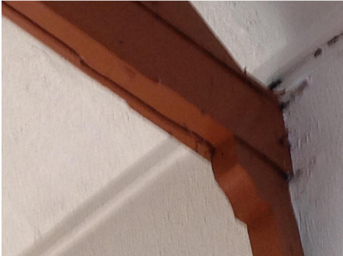
Image 6: Shows cracking in roof joists.
