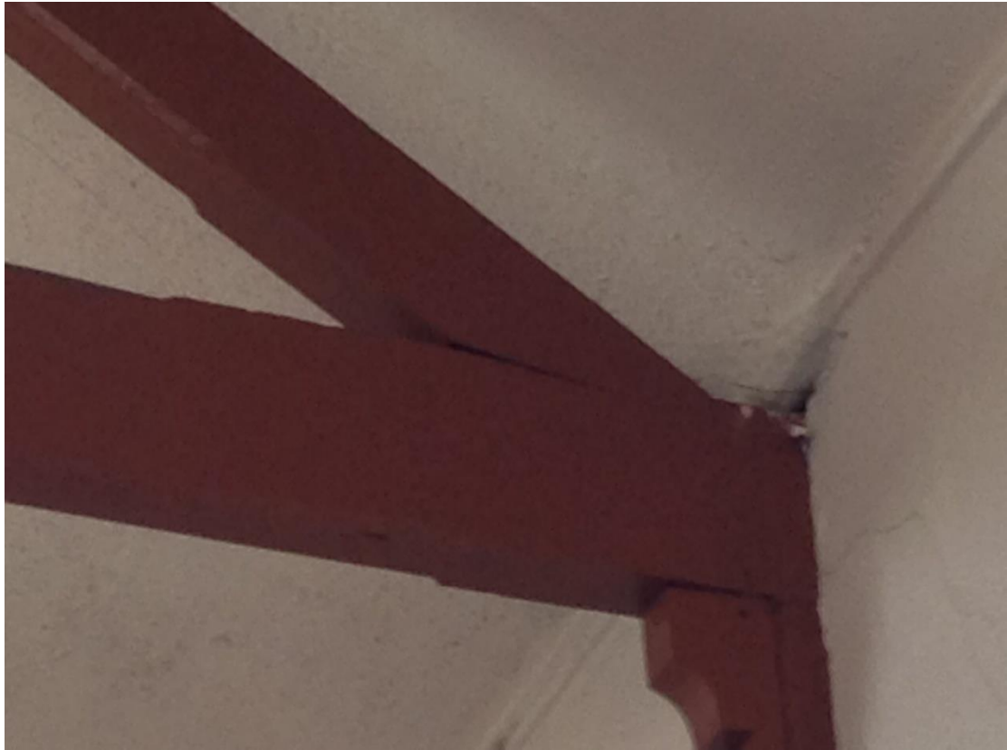
Image 4: Joist showing signs of movement and spread.
