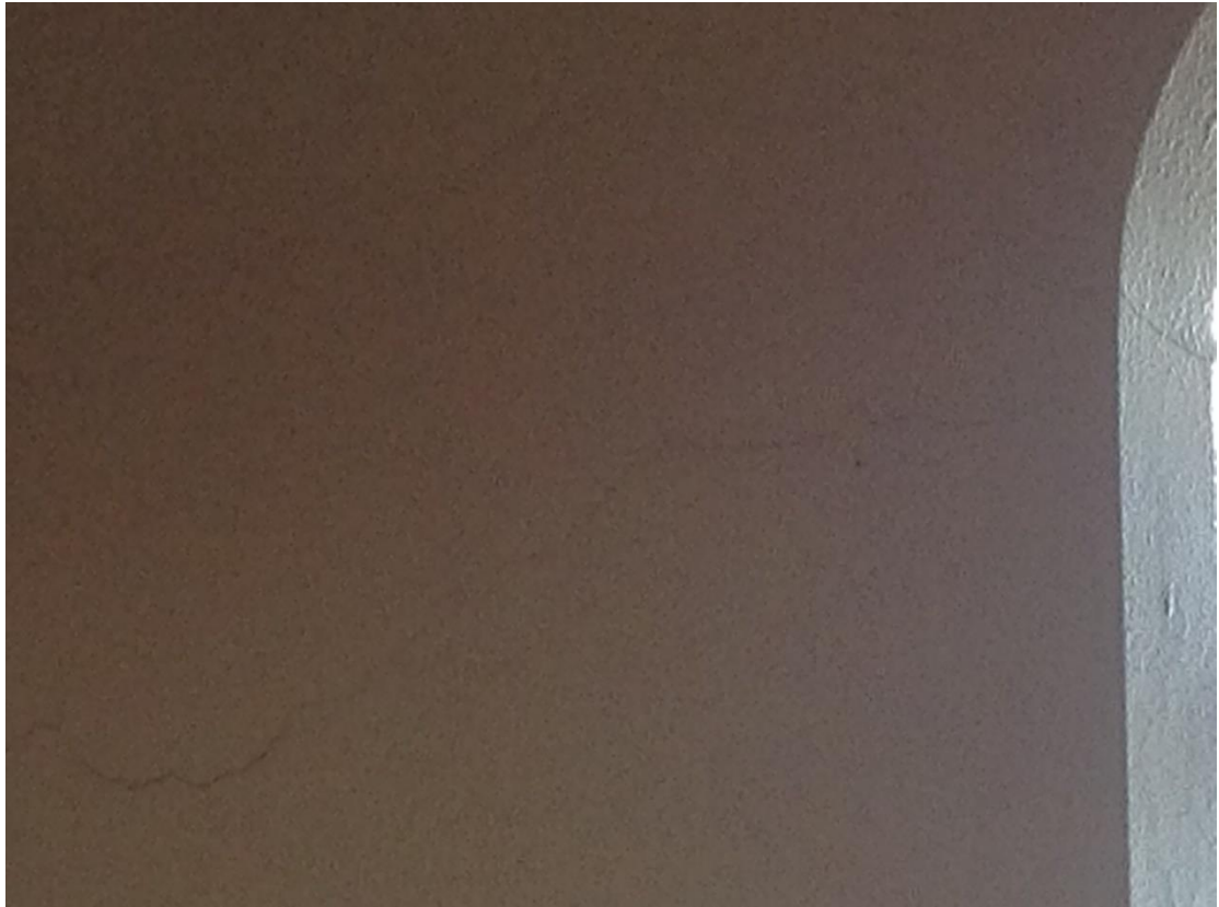
Image 2: Shows gable end wall cracking.
